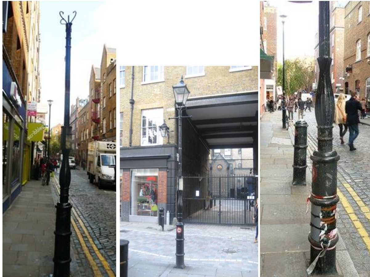
On narrow footways the road camber means lorries can hit the lantern (left two) and graffiti and loose covers are costly maintenance items. With façade lanterns such costs disappear.
